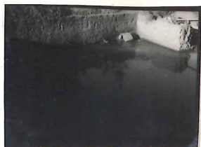
FLOODED BY OVERNIGHT POWER OUTAGE IN THE PUMPING SYSTEM
